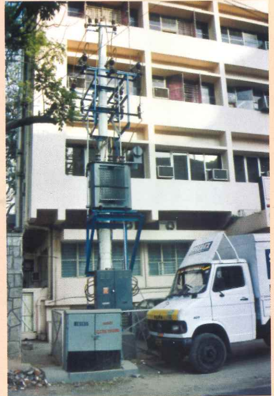
Single pole transformer in Bangalore
