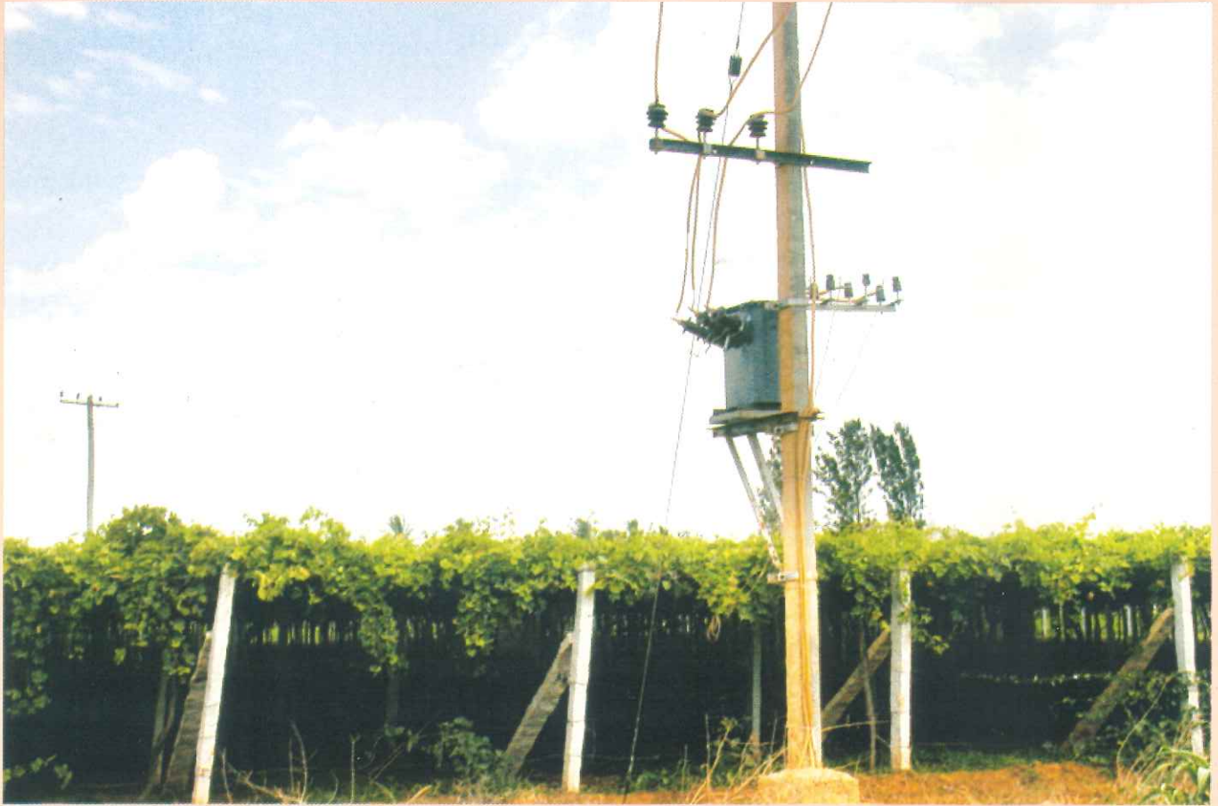
Single pole transformer ( Rural)
