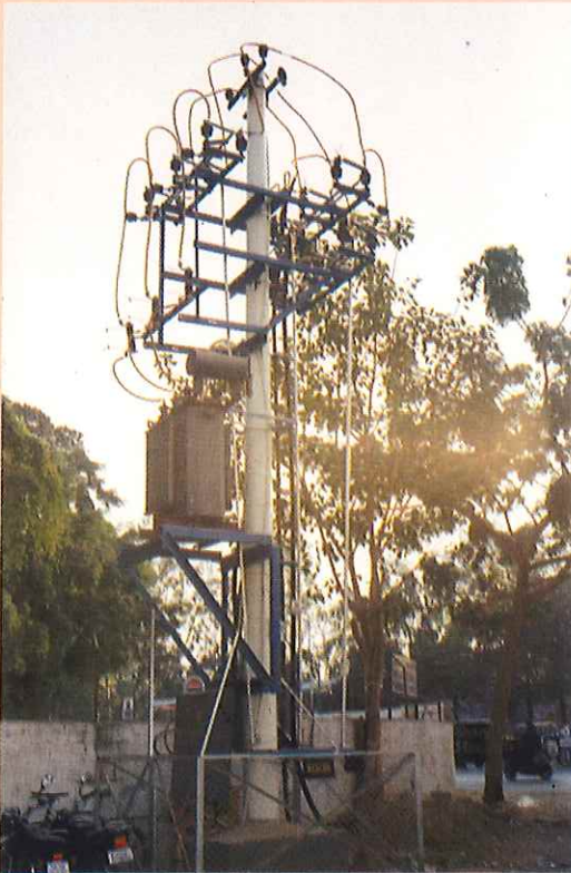
Single Pole Transformer in Bangalore city
