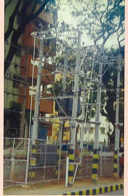
Conventional type transformer in Bangalore City
